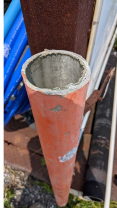
1" inch service lines
