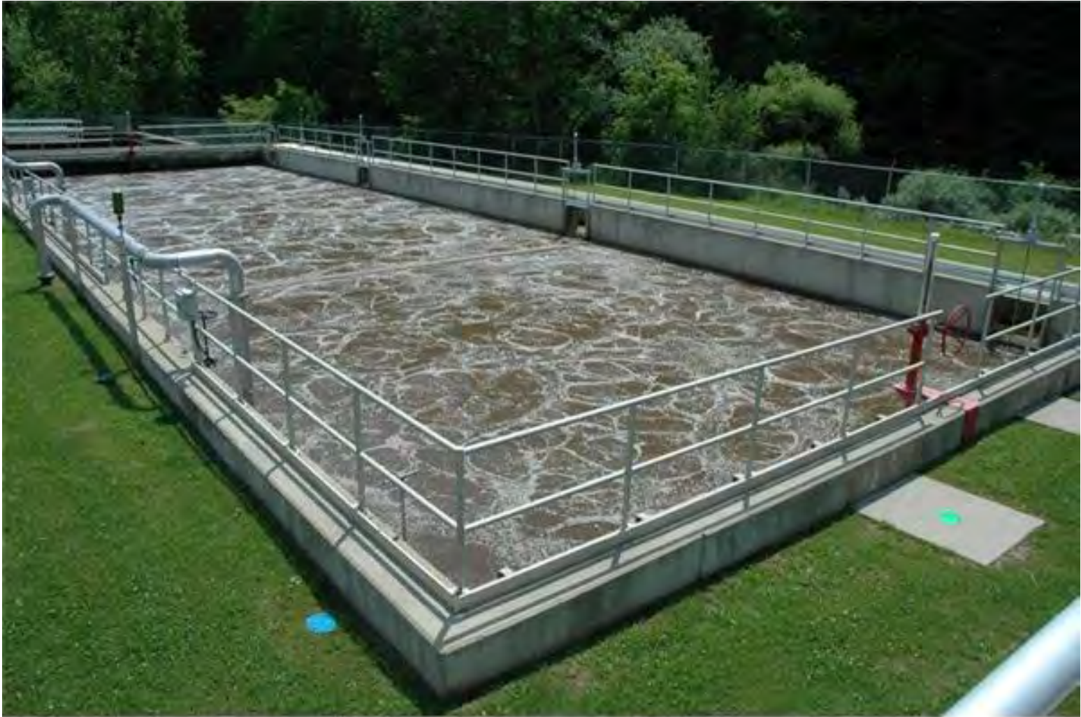
Activated Sludge Aeration Tank
