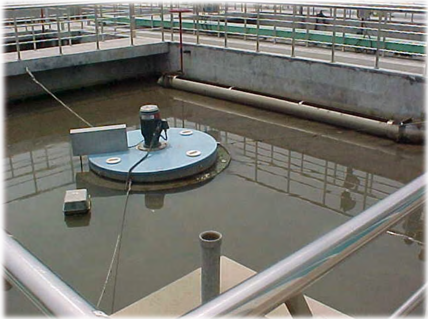
ANOXIC SELECTOR BASIN
